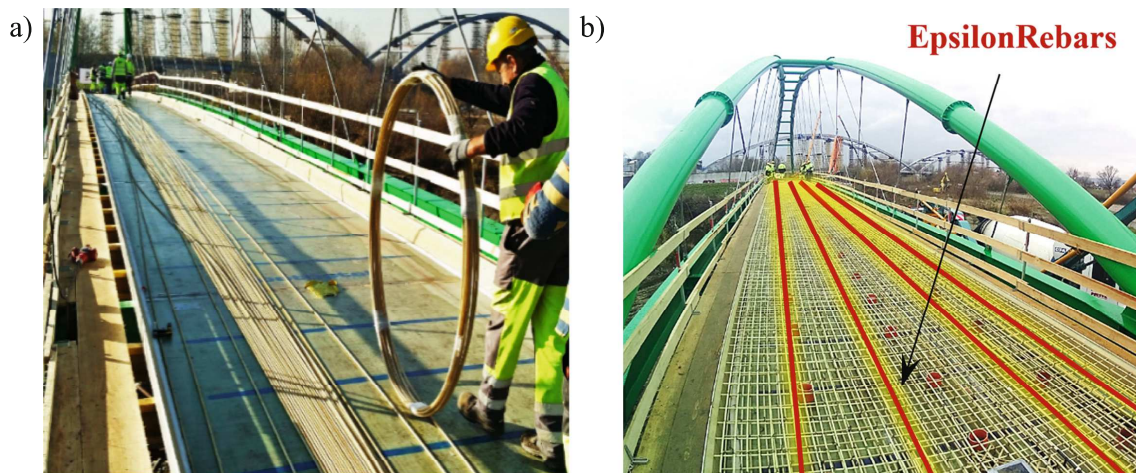
Fig. 7. a) Installation of DFOS composite EpsilonRebar sensors within composite deck panels, b) view of the composite reinforcement and EpsilonRebars just before concreting.
