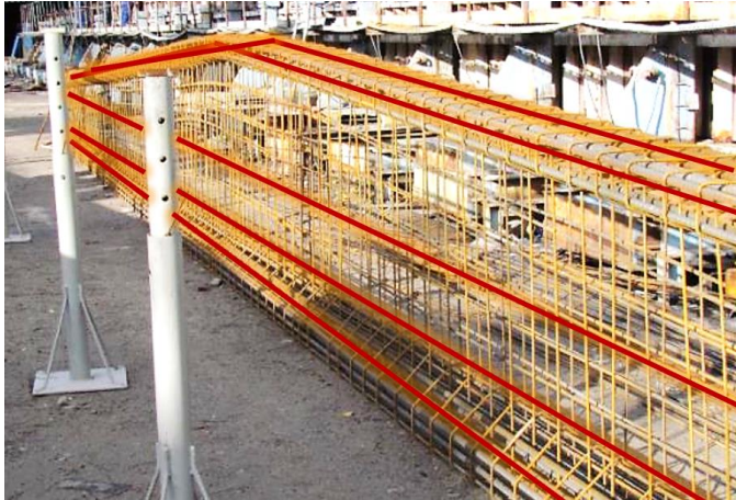
Figure 8. Installation of EpsilonRebars to the existing reinforcement of smart prestressed-concrete girder – side view
