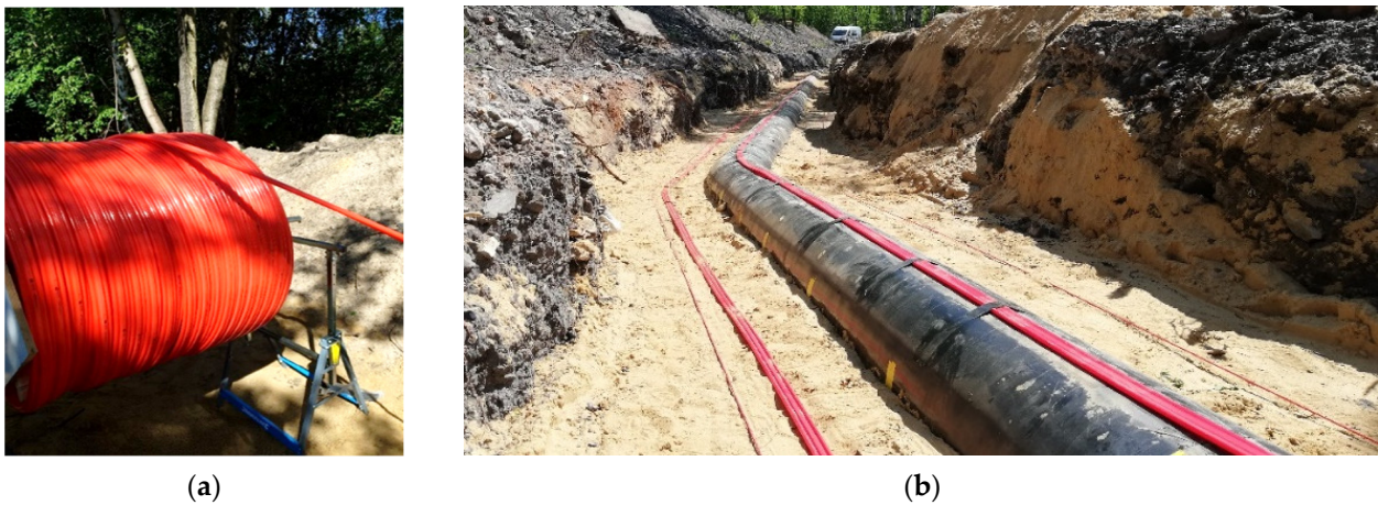
Figure 30. Gas pipeline equipped with 3DSensors: (a) delivery on site in the coil; (b) view of the installed sensors.
